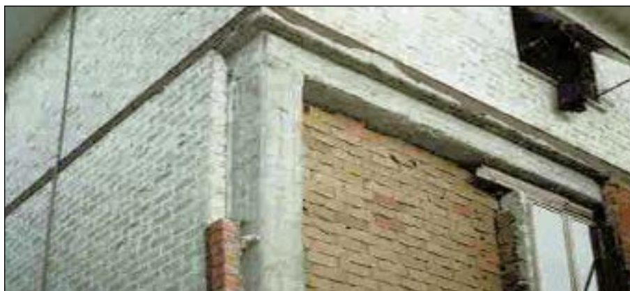
Figure 10. Example of dissymmetries in the infill panels (AeDES Manual).
